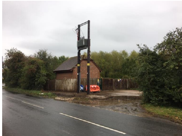
Raised substation at Burgess Bank, Yalding
